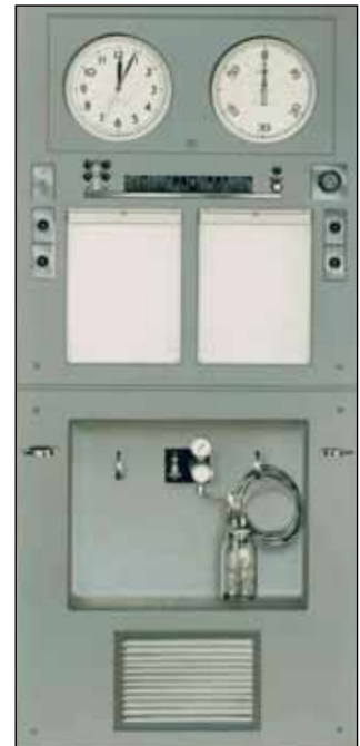
1972 Post Glover Isolated Power Panel
